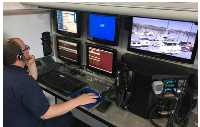
Above – Corey Hostetler, Assistant Supervisor uses remote connections to CAD and Harris radio systems to remotely dispatch Chester County Field agencies from the parking lot in Hershey PA.
